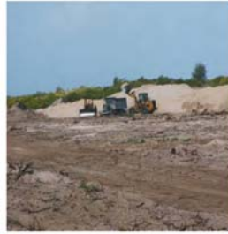
Figure 32. Ongoing sand mining near Palmetto Point.
